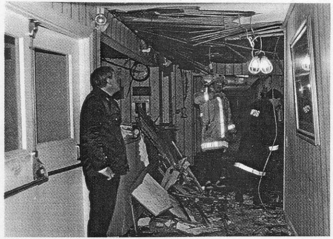
Explosion and fire damage in the core area of the nursing center extended from the first floor to the third floor, shown here. Fire doors at left closed automatically.
